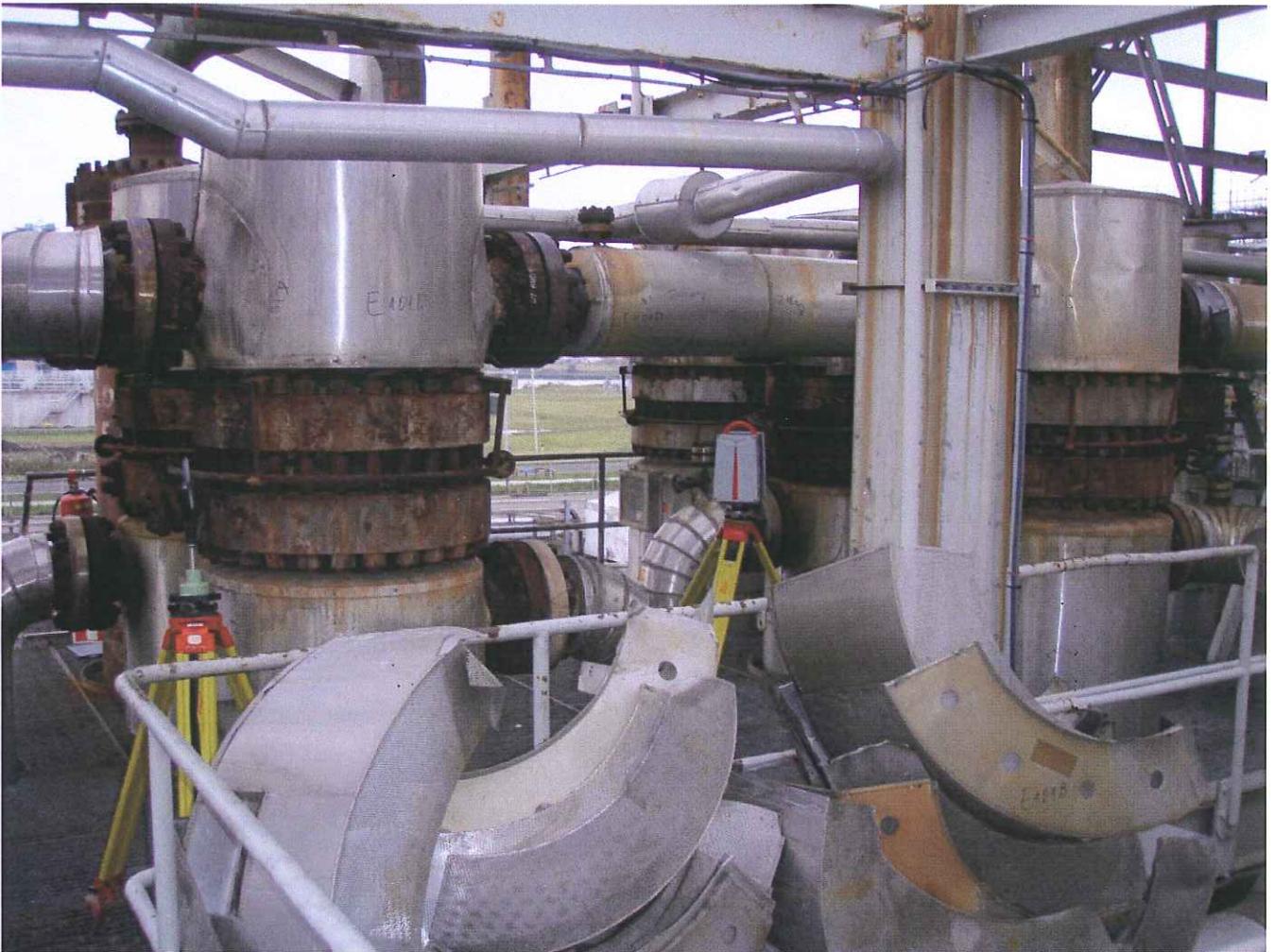
Case: Shell Pernis - Measuring the thermal expansion of heat exchangers
